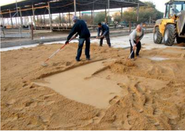
1 Spread the sand inside the steel tank boundaries uniformly to achieve a 10cm layer
