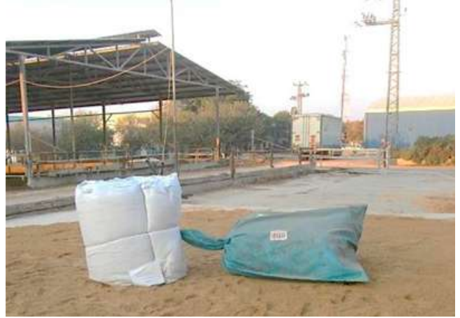
2 Position the protection textiles and tank liner inside the steel tank boundaries
